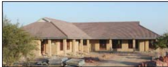
A home similar to this is being constructed in South Africa for AIDS-affected orphans with funds raised by Baptists for Life.
